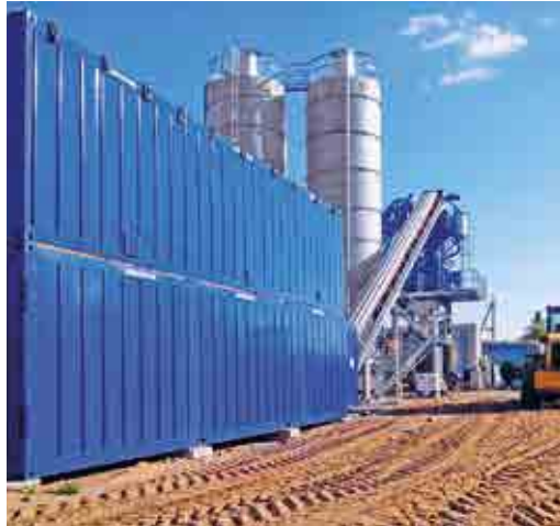
^ Semi-Mobile Batching Plant Type MCM
